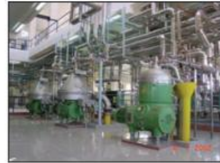
A piping network in an industrial facility.
