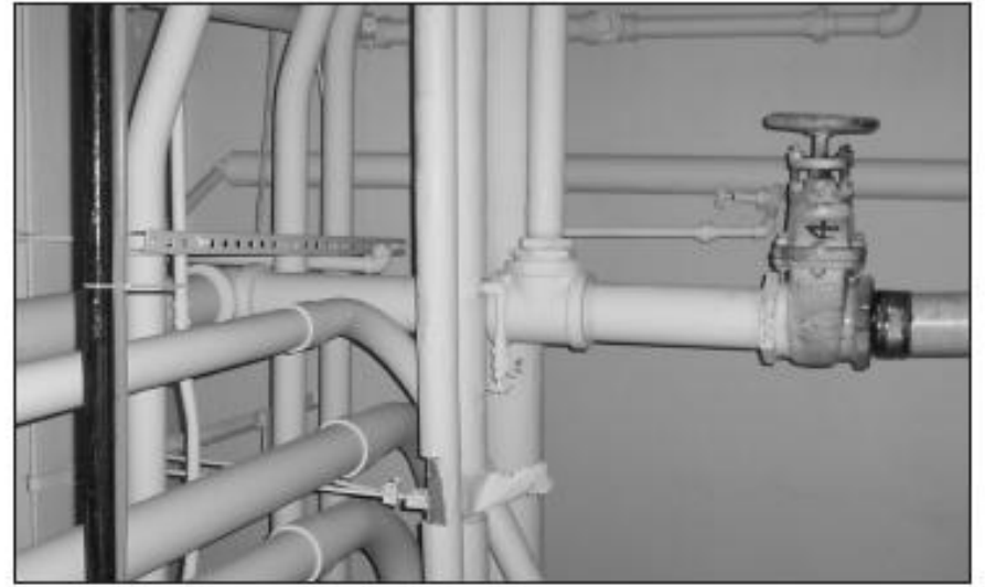
Piping and plumbing systems
